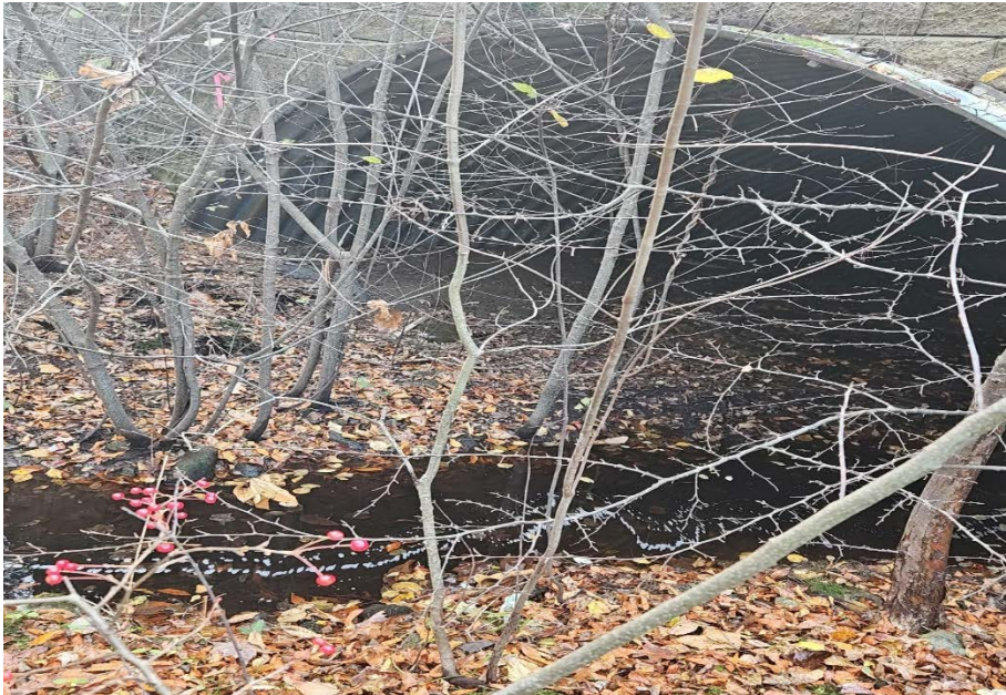
Photo #1: General view of culvert on northern side of Forest Ridge Drive with common winterberry ( Ilex verticillata , FACW). Photo taken on November 7, 2023, by Hancock Associates staff scientist.
